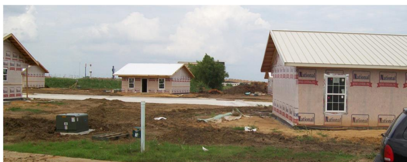
Homes being built by the Choctaw Nation in Durant, OK, provided by Southern Plains Office of Native American Programs staff, 2017 report Housing Needs of American Indians and Alaska Natives in Tribal Areas
